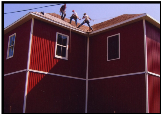
Maintenance, always... 2006 LFP 055
